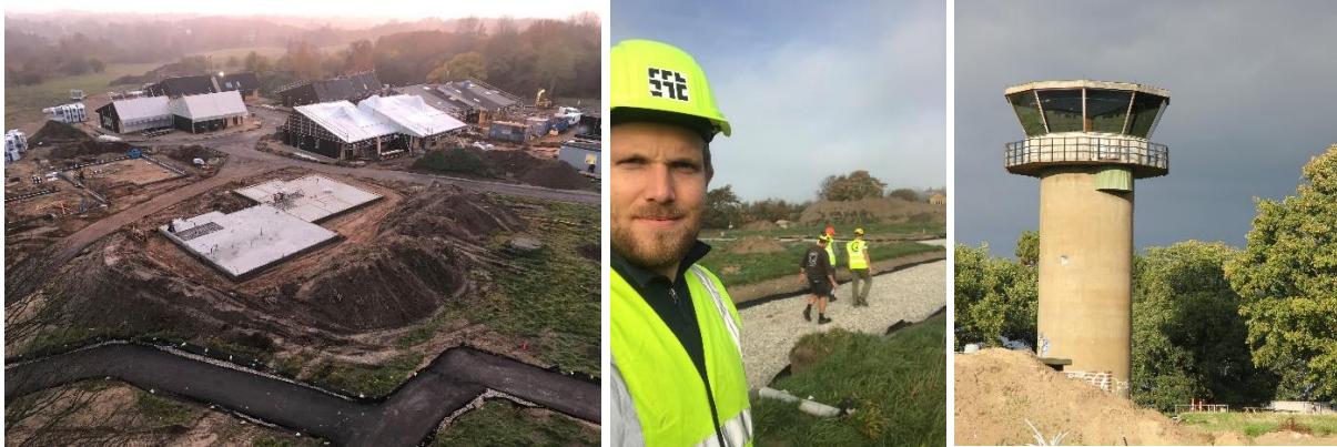
Figure, from left to right: The 10 first houses during the 2018-fall; Claus coordinating construction works with the contractor; The former NATO control tower that is now a part of the shared facilities in the project.
